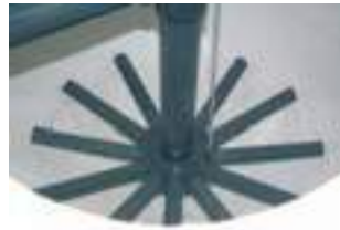
Collector arms detail
