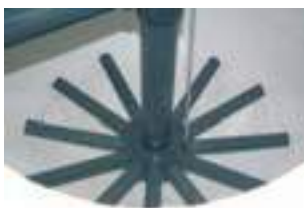
Collector arms detail
